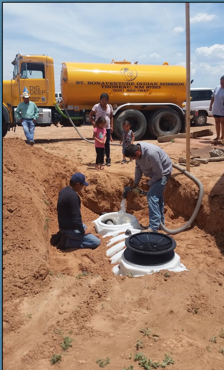
Dig Deep/Navajo Water Project crews fill a 1,200-gallon cistern at a home on the Navajo Nation. It's part of a self-contained system that brings potable water to families that lack indoor plumbing.
